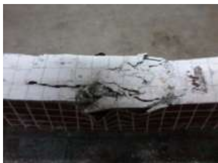
Figure 13. Failure pattern by crushing of concrete in pure bending
